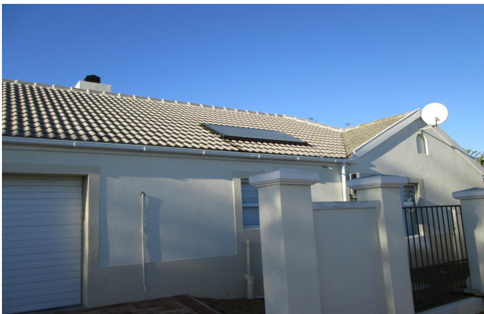
Figure F1 Example of an acceptable installation of a solar heating panel
